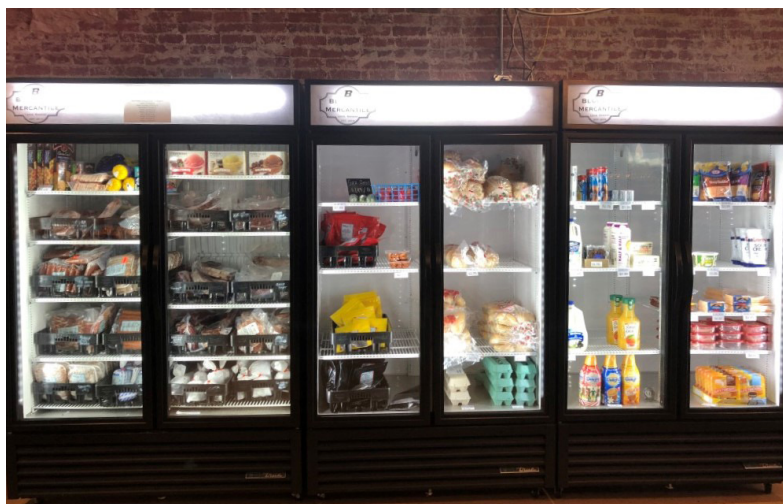
Coolers at the Bluestem Mercantile.
